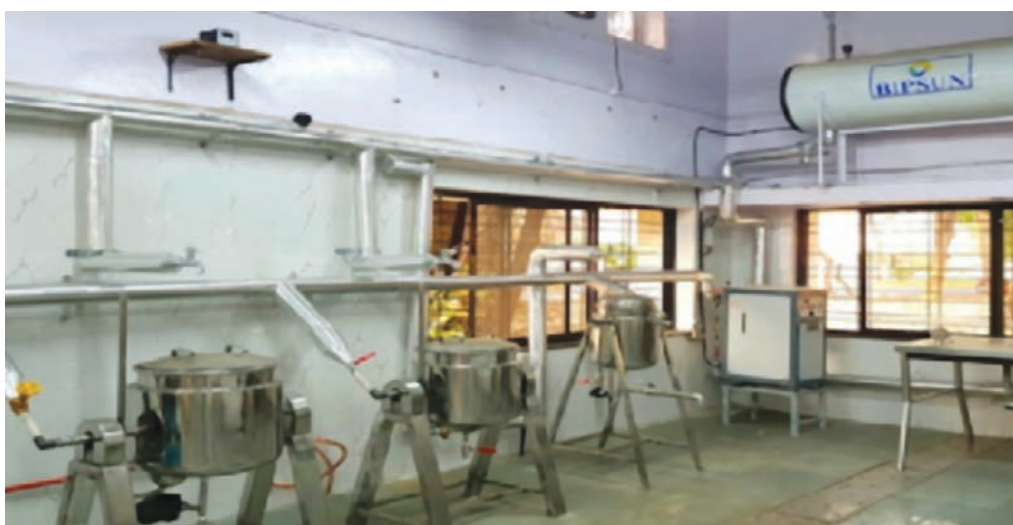
Eco-Friendly Solar Cooking System installed at CSIR-NCL canteen
