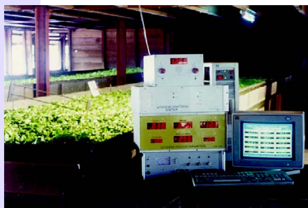
Withering Trough Automation System at Gulma Tea Estate
