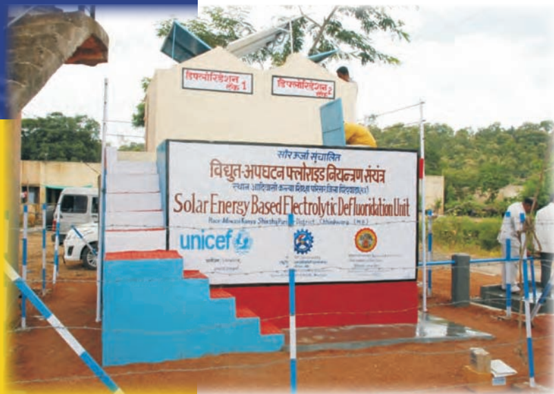
Solar power based EDF plant at Adiwasi Kanya Shiksha Parisar, Chhindwara
