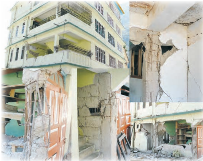
Figure 4: Typical failure of RC buildings in Chungthang
