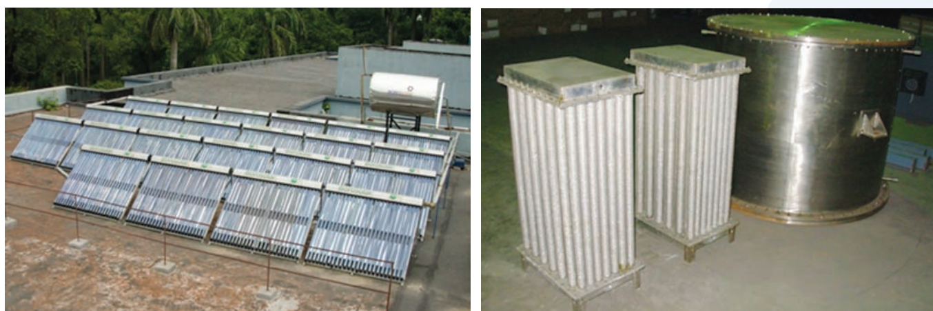
Fig. 5. Solar Water Heating System and Sorption Heat Exchangers at CMERI
