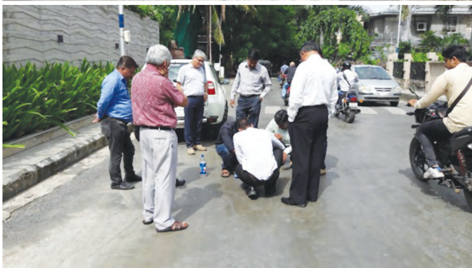
Stakeholders of the technology (left) and Skid Resistance Measurement on CGBM section after two months of laying (right)
