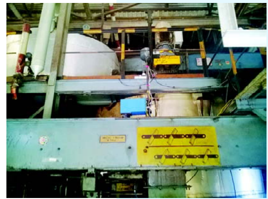
Fig. 2: Copra moisture sensor installation at Marico
