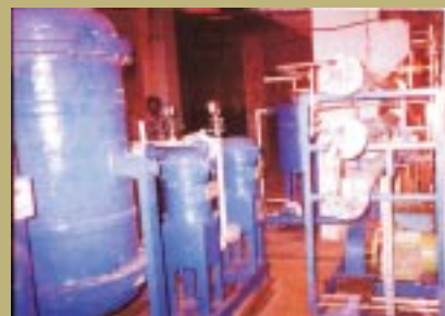
A view of CFCL Plant at Haldia, West Bengal, based on IICT technology
