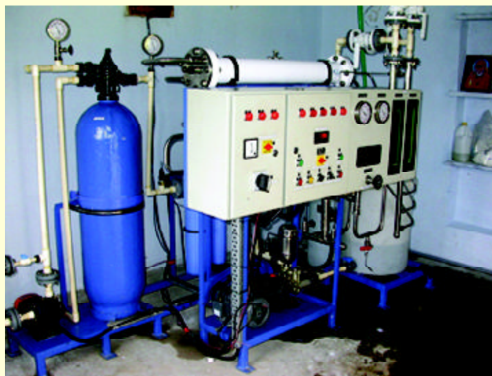
A view of reverse osmosis pilot plant, designed and installed by IICT, in Nalgonda District
