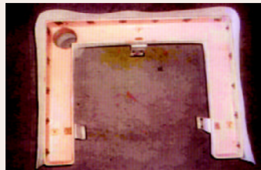
Inner view of FRP hopper
