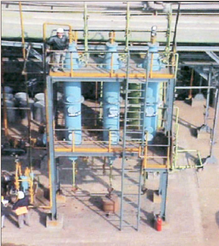
Aerial view of pilot plant for bio-deodorization of industrial emission containing pyridine at M/s Jubilant Organosys Limited, Bharatiyagram, Jyotiba Fule Nagar, Uttar Pradesh
