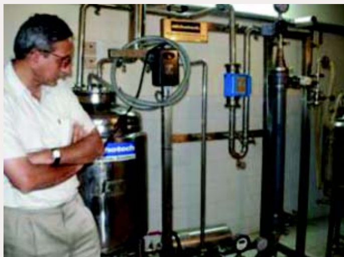
Neera filtration facility at GNMDTC, Dahanu
