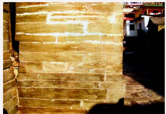
Fig. 5 : Indication of Settlement and tilting
