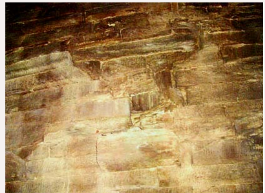
Fig. 4 : Indication of water seepage
